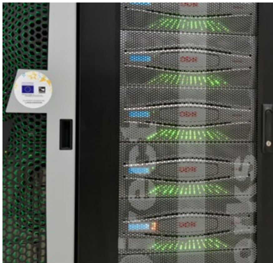
The DATARMOR supercomputer (located at the Ifremer Brittany Centre), with its impressive data storage capacity and computing power. © Olivier Dugornay - Ifremer
